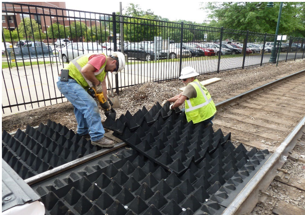
Figure 2. Anti-trespass panels installed at a grade crossing in Fayetteville, AR. Image Credit: Volpe Center
